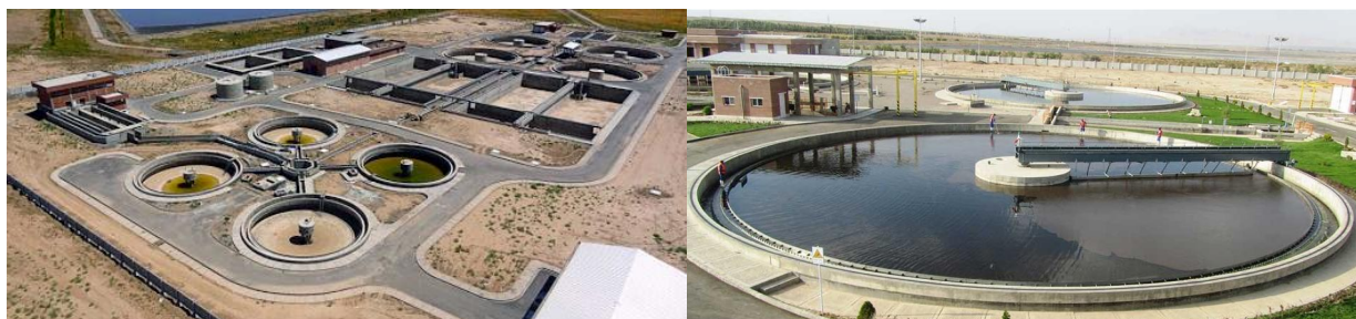
Wastewater Treatment Plant, Mashad
