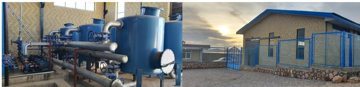
Water Treatment Plant, Sarajooy-Maraqeh
