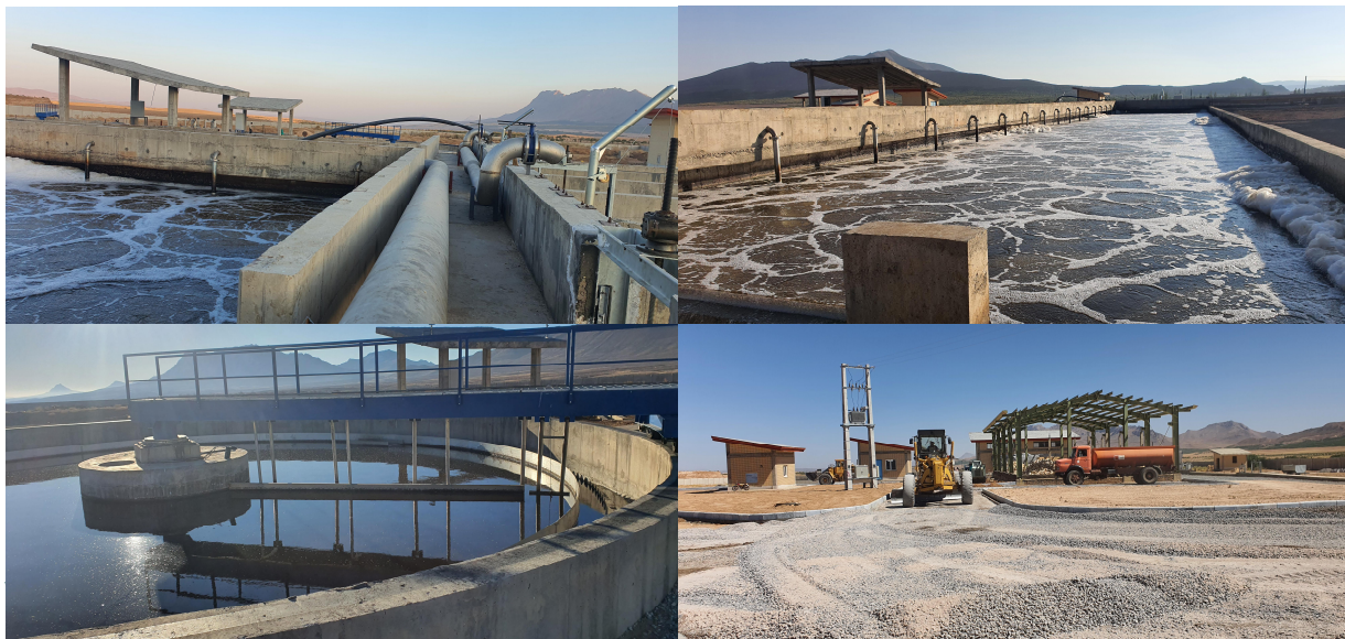
Wastewater Treatment Plant, Ben City-Charmahal Province
