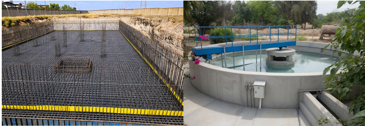
2500m3 water storage Tank, Sepehr Industrial Park-Karaj
