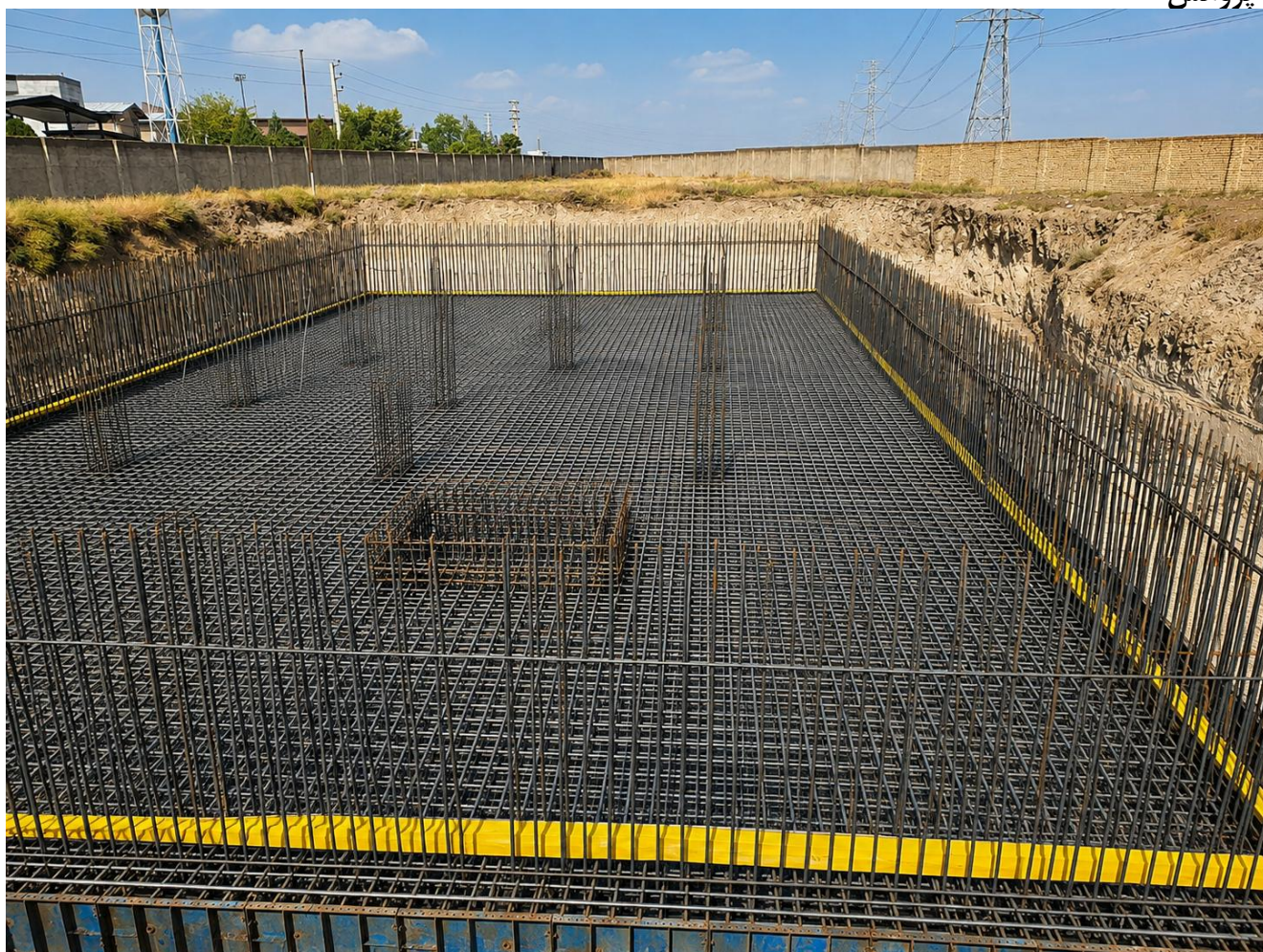
250cubic meter water storage tank, sepehr industrial park Figure
