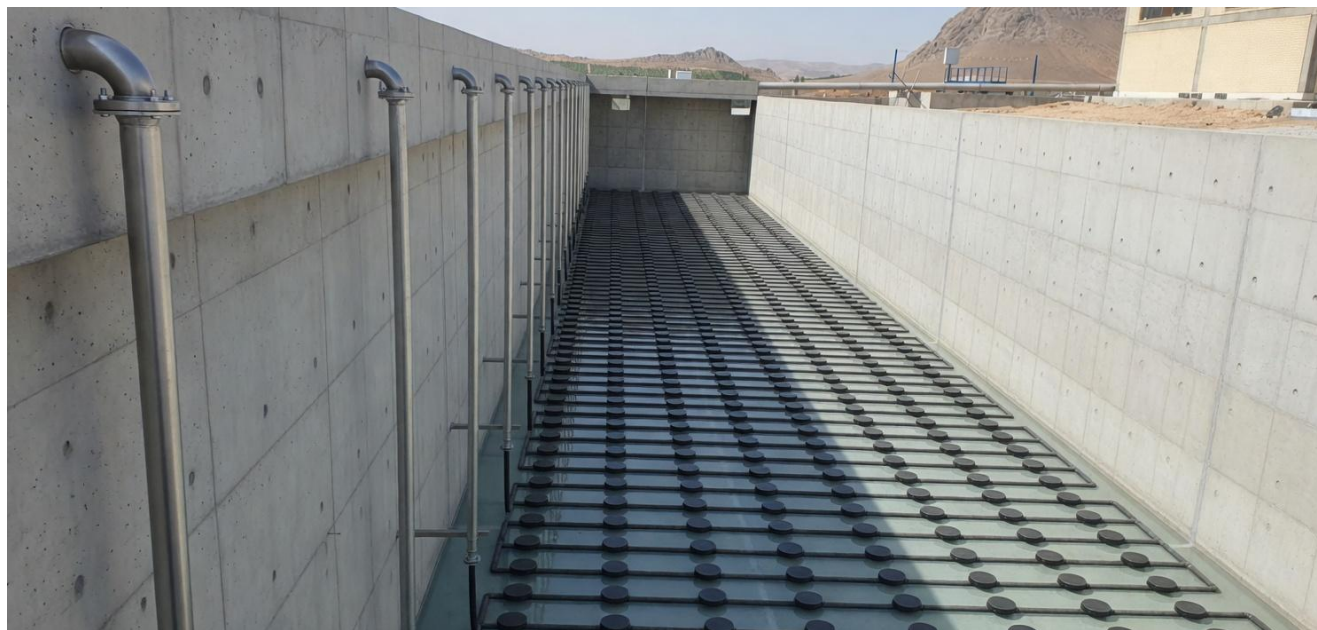
Figure ۴ Wastewater Treatment Plant, Ben-Shahrekord
