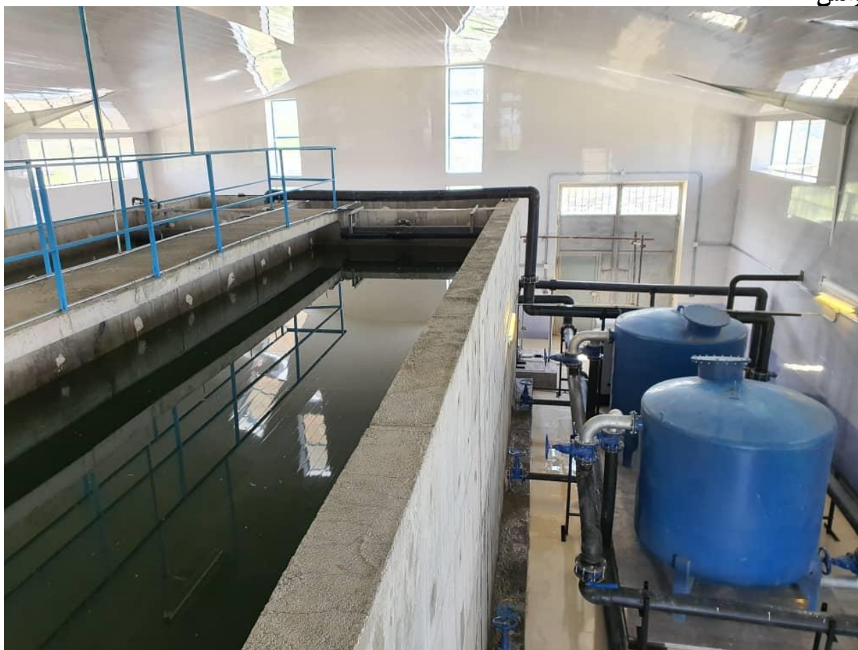
Figure ۲ Water Treatment Plant, Qolyan-Sanandaj
